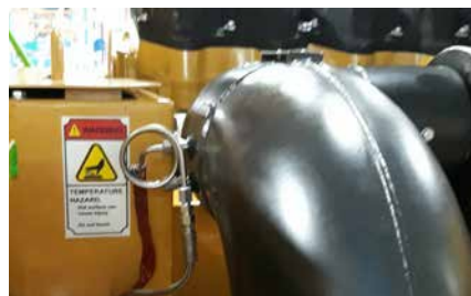
Custom pipe fabrication with pipe-mounted probes
