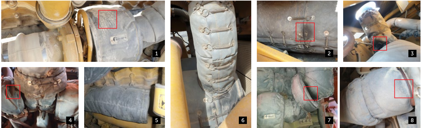
ABOVE Residual dirt build-up and low-level soot are typical (1,2,6). Investigate prominent soot on blankets for engine pipe leaks (3,7). Eliminate gaps and refit blankets (8) for a snug-fit and maximise coverage (4). Monitor blanket condition during ongoing maintenance.
