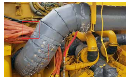
Add blankets to protect high voltage lines against contact with hot exhaust surfaces
